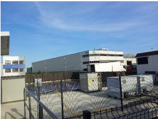
Friselva WWTP biological reactor
