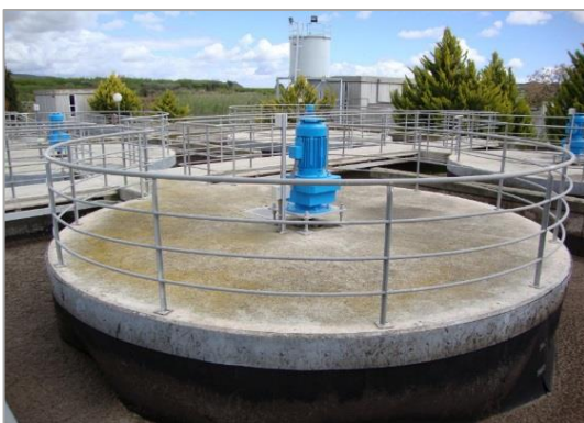
Aeration system (turbine) of Cehegín WWTP biological reactor
