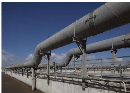
Air supply to the biological reactor of Barcelona Baix Llobregat WWTP
